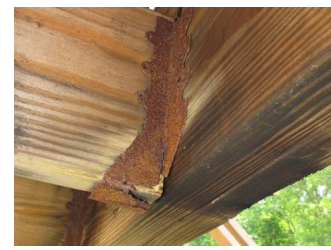
Loose or corroded fasteners: Tighten fasteners, replace rusted/corroded fasteners
