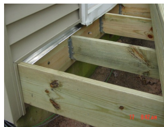
Flashing: Check to make sure it is sound and firmly in place
