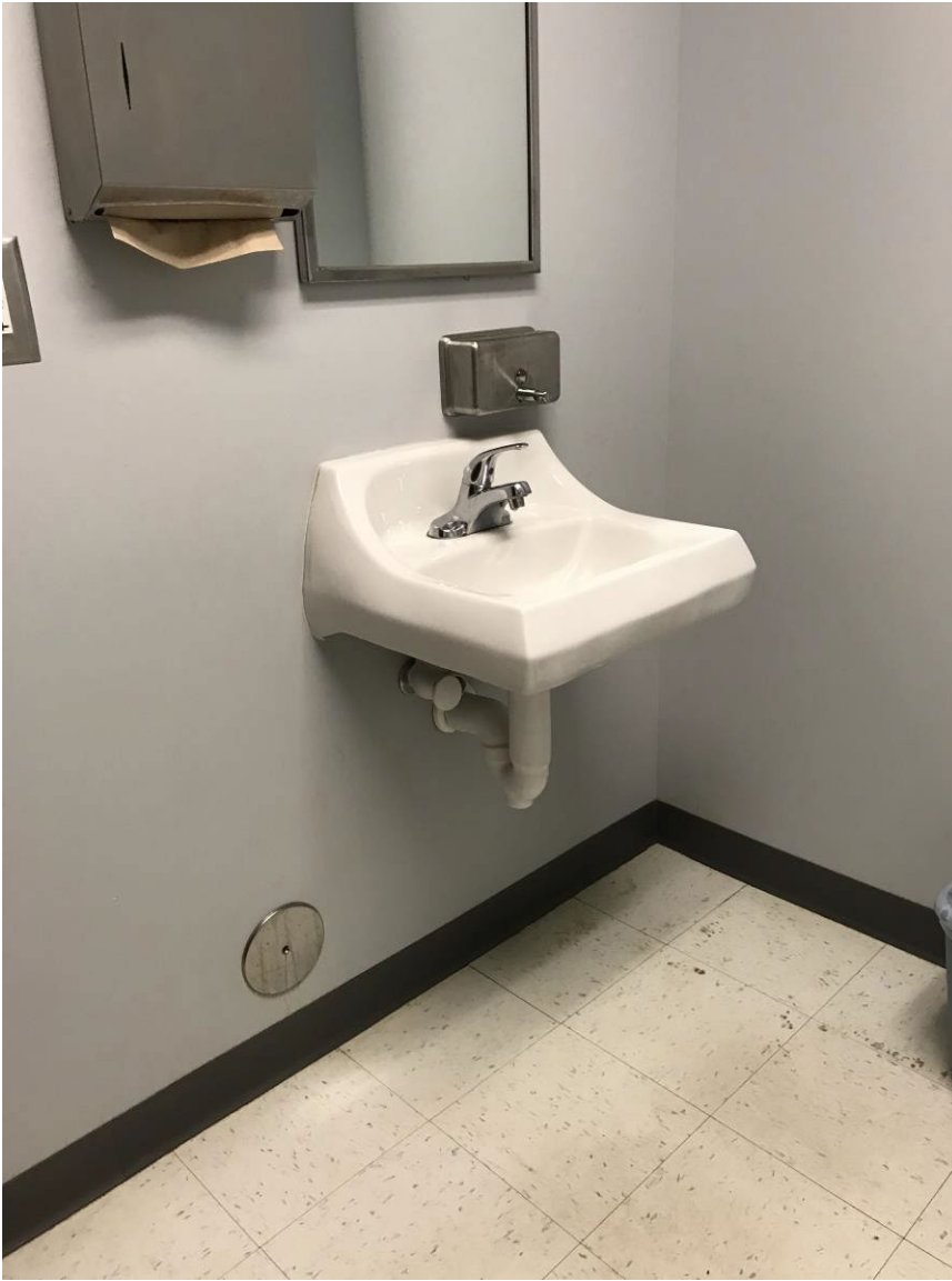
Sink with pipe protection
