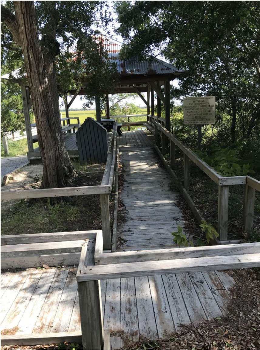
Ramp to covered picnic area. Path to ramp needs to be non-slip surface
