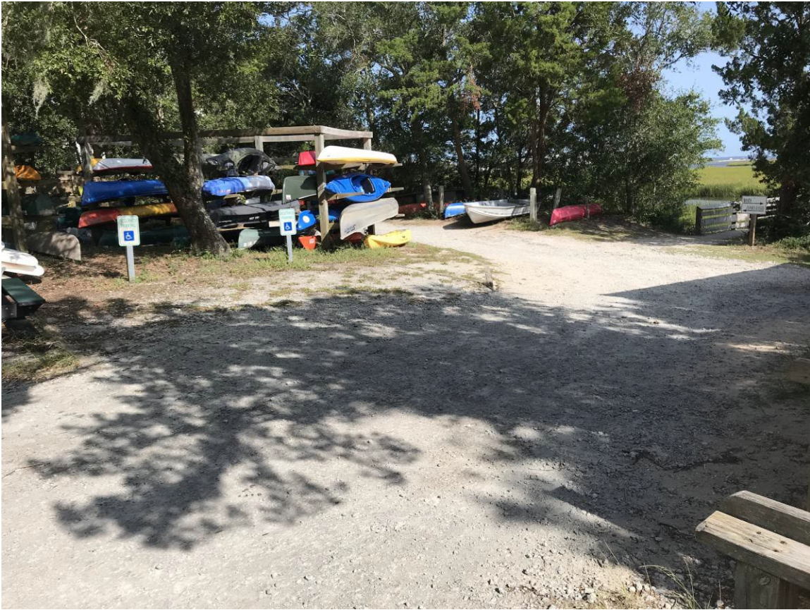
Accessible Parking. Needs to be non-slip surface
