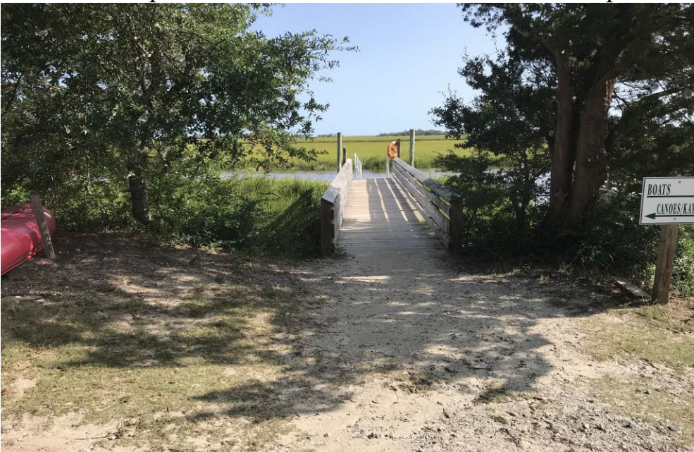
Path to dock. Needs to be non-slip
