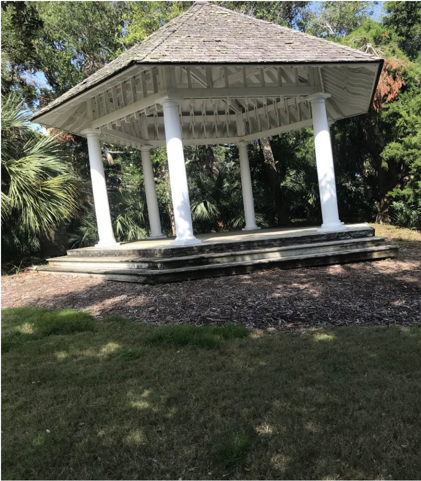
Raised gazebo that a ramp is recommended to make it accessible.
