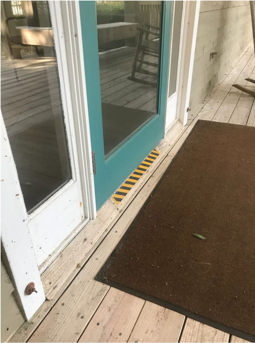
Threshold has too much change height
