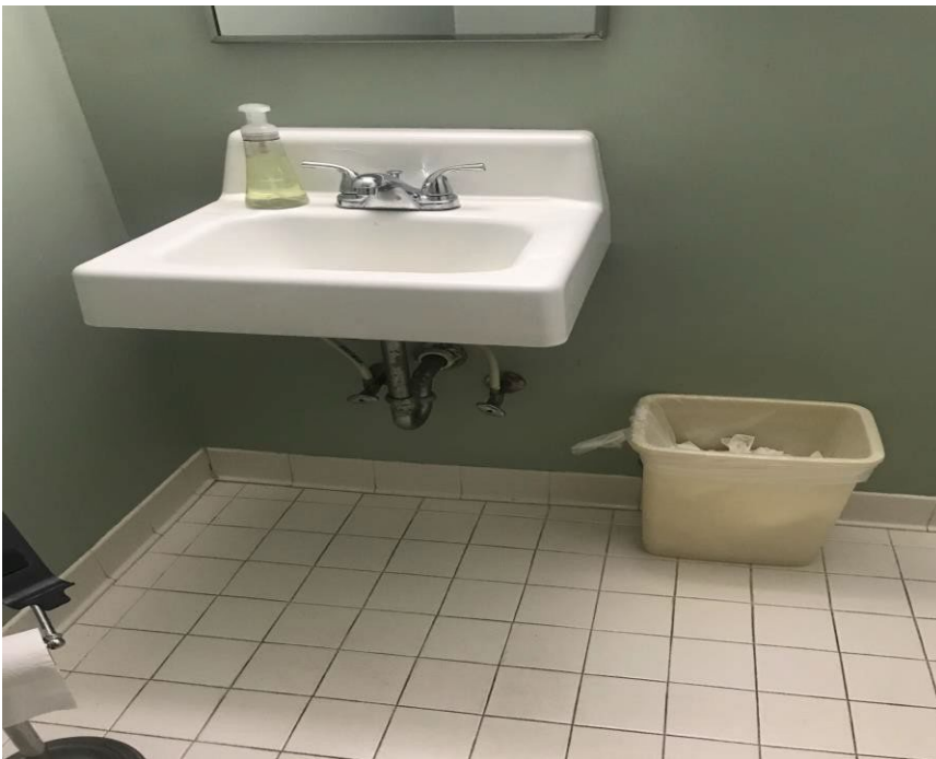
Pad/insulation needed to cover pipes under sink
