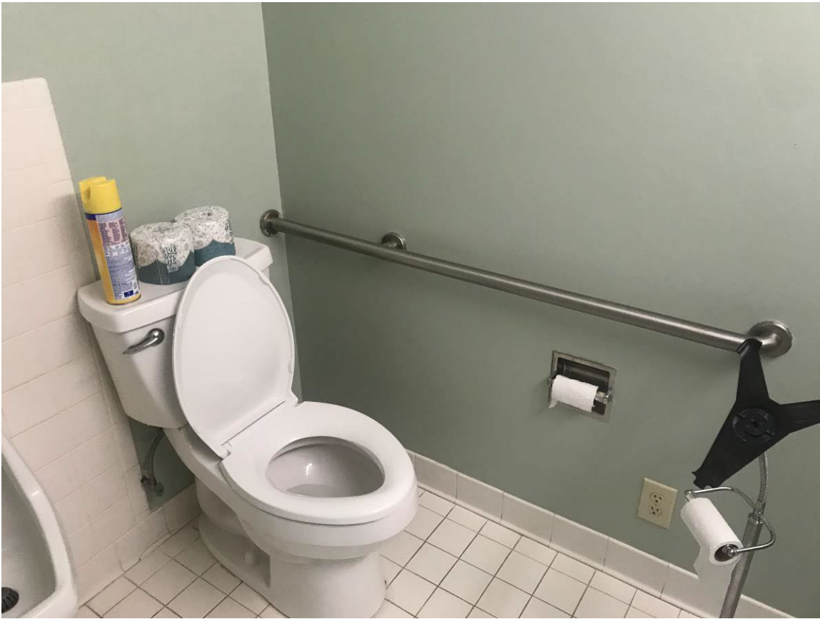
Missing grab rail at rear of toilet
