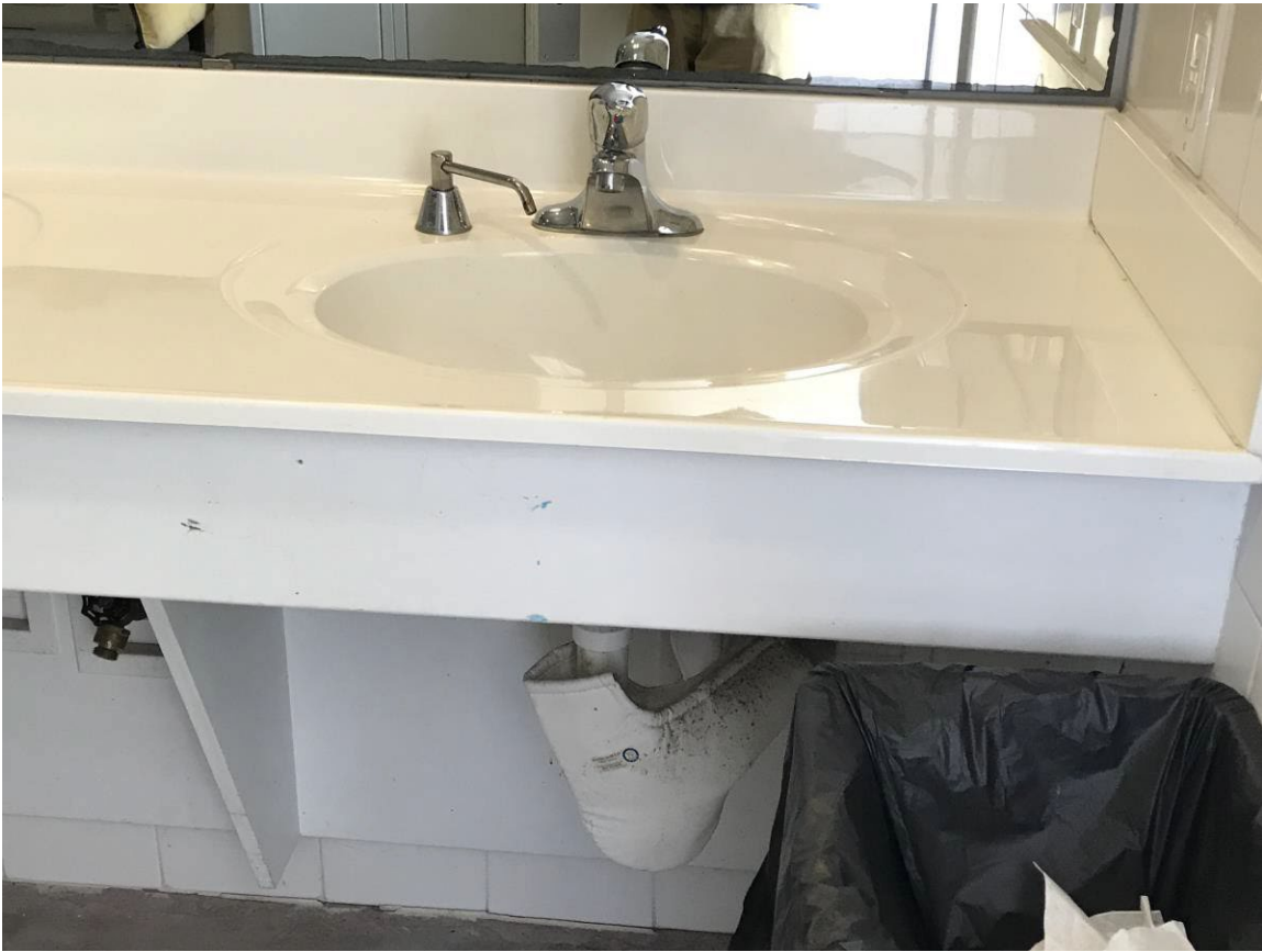
Sink with pipe protection
